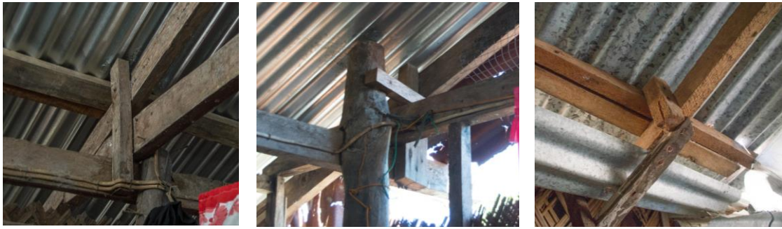
Figure 12. Examples of effective timber connections in the roof. Source: Pictures by Erika Palmieri
