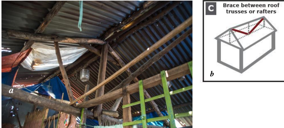
Figure 13a. Example of strong brace between roof trusses. Source: Picture by Erika Palmieri, Figure 13b. Technical drawing of roof brace from Shelter Cluster guidelines, Source: Shelter Cluster Philippines guidelines
