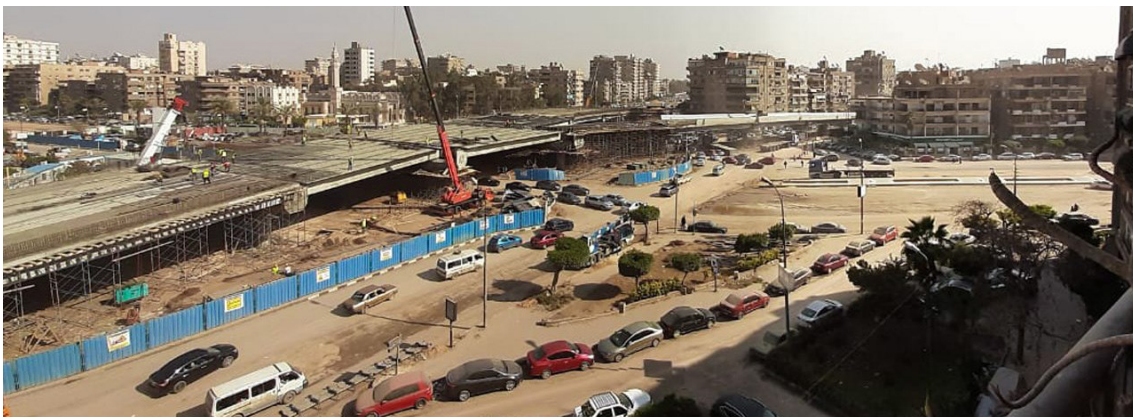
Figure 8 Above shows a before photograph of the roundabout at the intersection of Othman Ibn Affan and Abdelaziz Fahmy in Heliopolis. Source: Arafa, E. (date unknown).
