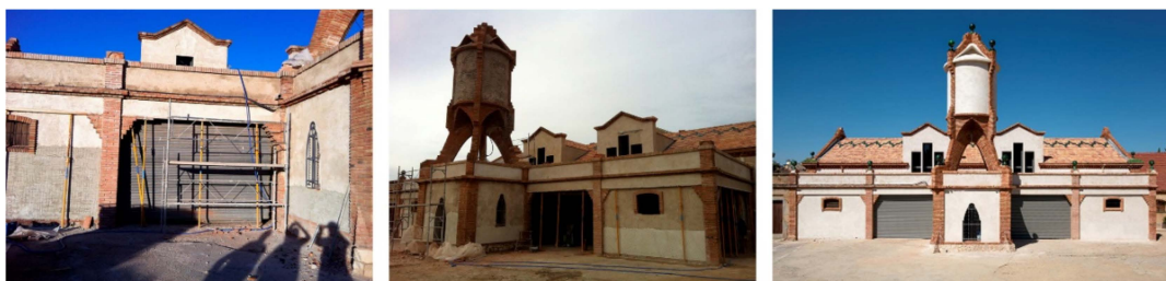
Figure 26. Back façade during restoration ( left and center ). Back façade after restoration ( right ).
