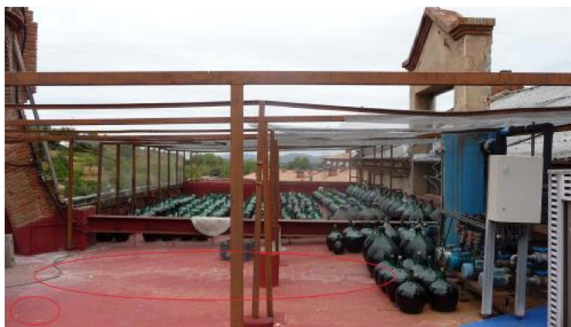
Figure 19. Deterioration of the surface of the flat roof.
