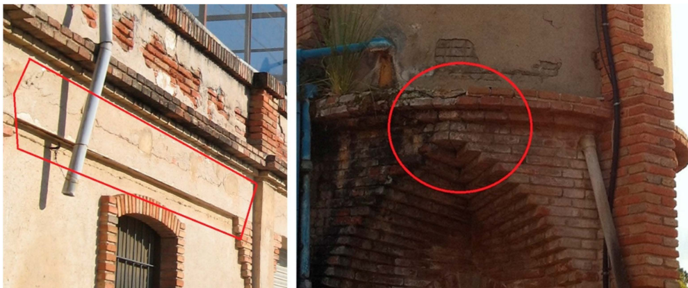
Figure 16. Cracks in the top part of the façade and in the water tank.
