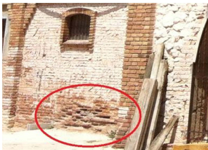
Figure 13. Deterioration of the base of the façade.
