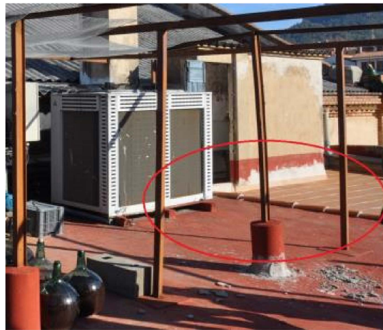
Figure 20. Discordant paving on the flat roof.
