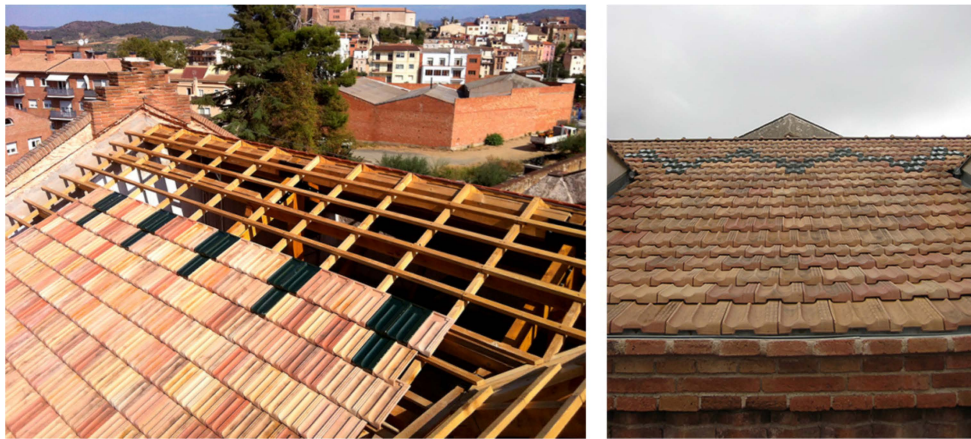
Figure 29. Roof of the wine-production-nave during restoration (exterior detail of tiles) ( left ). Roof of the wine-production nave roof after restoration (exterior detail of tiles) ( right ).
