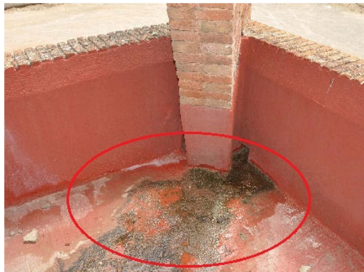
Figure 18. Dampness on the surface of the flat roof.
