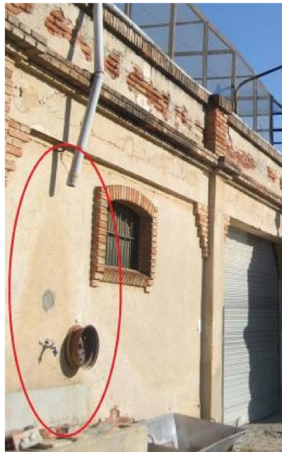
Figure 15. Dampness on the façade.
