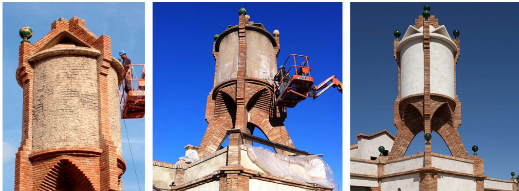
Figure 25. Water tank during restoration ( left and center ). Water tank after restoration ( right ).
