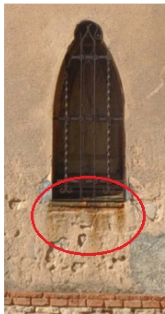
Figure 10. Rusting of the original bars of the windows.
