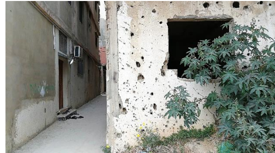
Figure 32. Houses in ruins: the living memory of the 2007 war Source: Author's archive.
