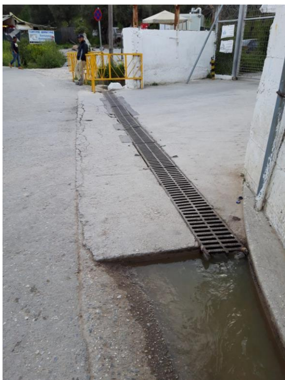
Figure 5: Open sewage flowing towards the entrance Image source: Interviewee Beni's archives
